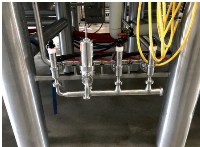
Feed gas collection manifold
