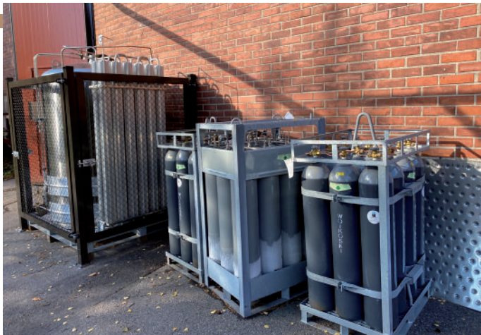
CO 2 storage tank delivered by Dalum along with CO 2 container bundles used during the startup phase (Fat Lizard, Finland)
